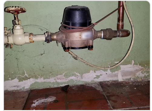
Water main and shutoff
