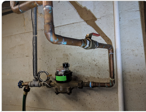
Water main and shutoff
