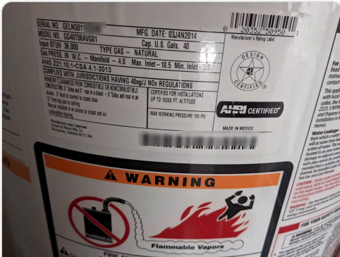
Equipment schedule · Water heater data plate
