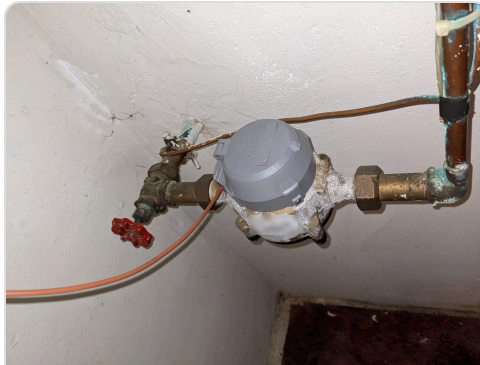
Water main and shutoff
